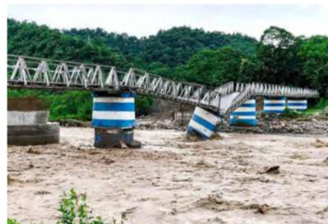
Disaster strikes: A video grab of a portion of the Dudiya iron bridge which collapsed in heavy rain in Darjeeling on Saturday night. ANI
