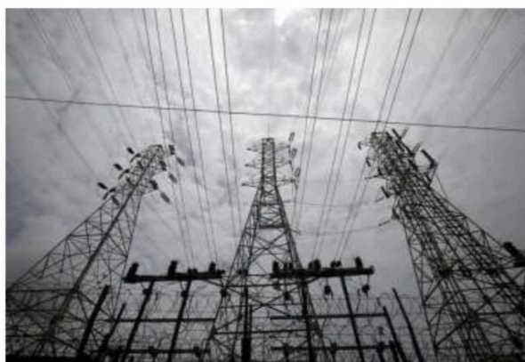
Power struggle: India's peak power demand has been hovering between 230 gigawatts and 250 gigawatts in the past week. REUTERS
